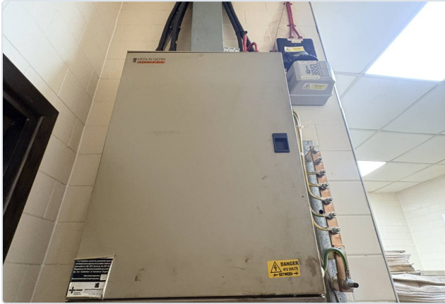
P1 — Distribution board, kitchen
