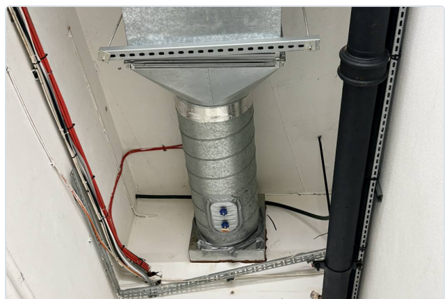
P6 — Extract duct riser
